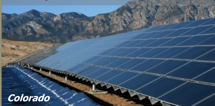
Solar array installed on landfill cap
