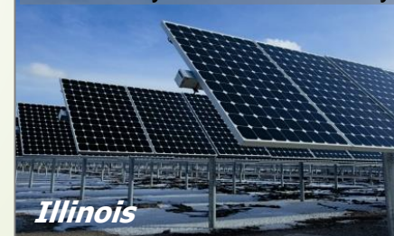
Solar array at former foundry
