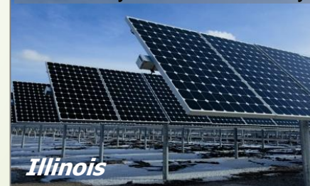
Solar array at former foundry
